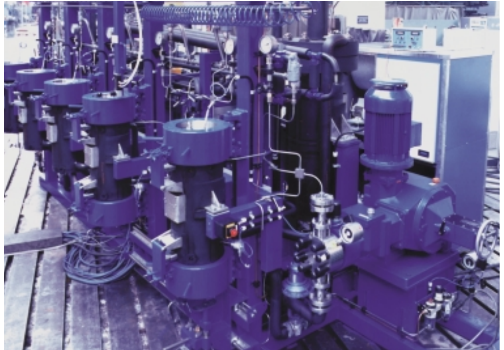
High pressure extraction plant with diaphragm metering pump EH1 (Company picture UHDE high pressure technology GmbH)
