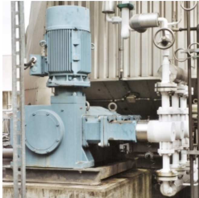
LEWA triplex plunger pump G3S in a CO 2 bottling plant
